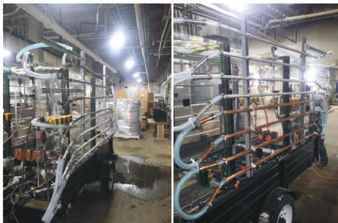
Figure 2 (left) and 3 (right). On the left, a pipe loop displaying PEX-A train (on top of pipe loop), Galvanized Steel train (top of loop wall) and Copper-K train (bottom of loop wall). On the right, a pipe loop displaying Lead train (top of pipe wall) and PVC train (bottom of pipe wall).
