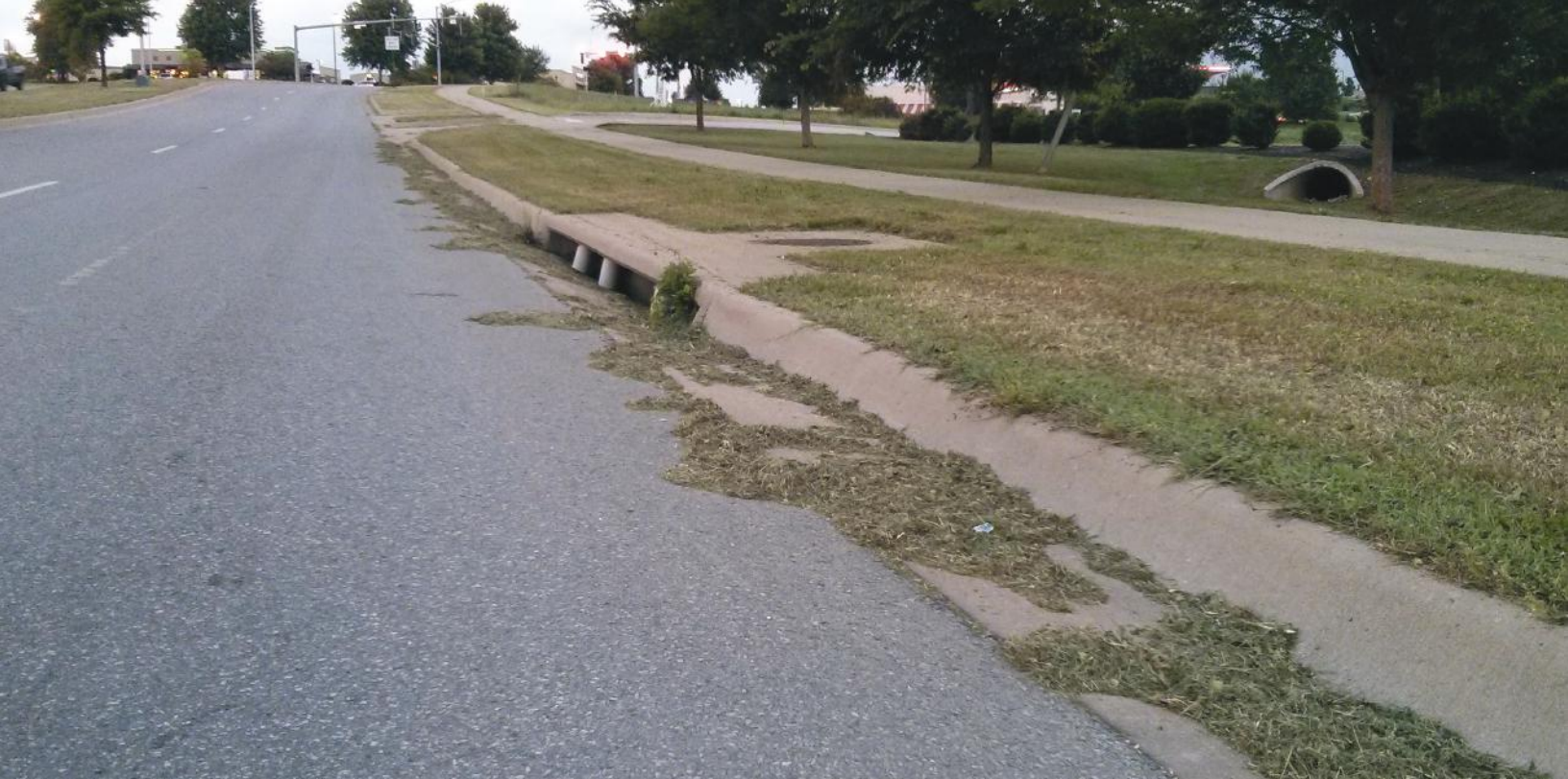
Image caption: Grass clippings on roads can be washed into the stormdrain when it rains, and can cause pollution in receiving streams.
